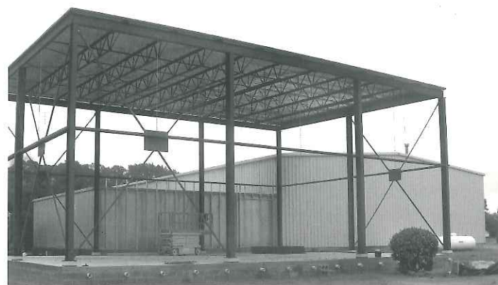
On the left is the frame of the 2,700 square-foot freezer. With pallets stacked four high, the usable freezer space is over 6,000 square feet.
